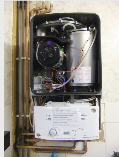
Lee Hagwood, New Boiler, CC BY NC
